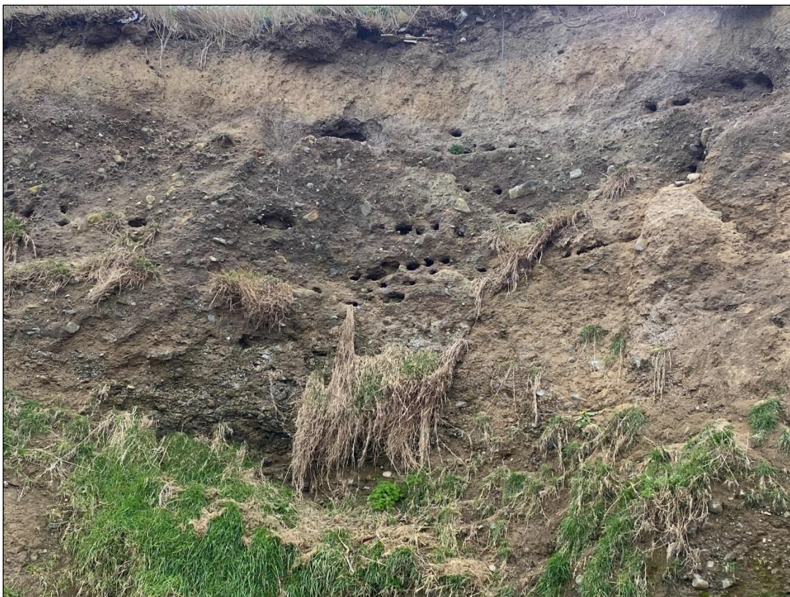
Figure D-2: Sand Martin burrows recorded in sea cliff adjacent to works area – 27-03-2025.
