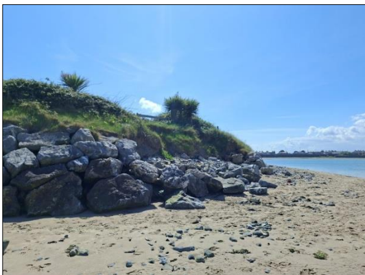
Photograph 3 – At the northern extent of the golf course looking south. Repair works required within the existing rock armour – [DR 06/05/2026]
