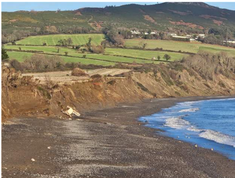
Photograph 8 – View looking north to Area I and J showing sections of cliff erosion – [Mc.B. 10/12/2025].
