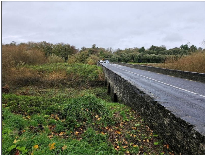
Photograph 6 – Area G of proposed MAC area; looking north at bridge [JMC 30 October 2025]
