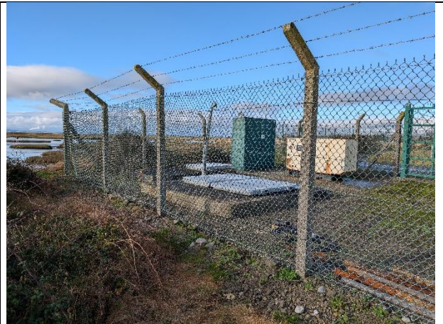
Picture 8: Pumping station at Area I, looking SW, RB
