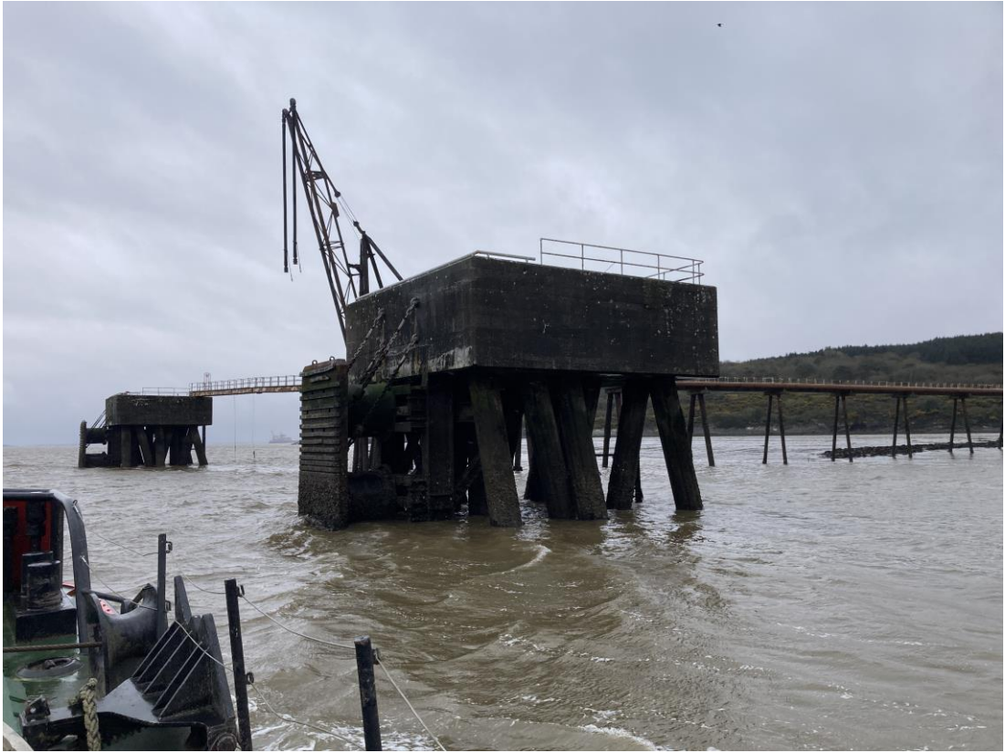
Photo 1 Existing disused and derelict oil discharging jetty and pipeline on trestle ashore (BMcD 26/03/2024).
